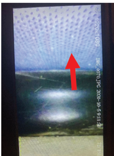
Endoscope view of cavity behind blockwork with breather membrane to OSB board
